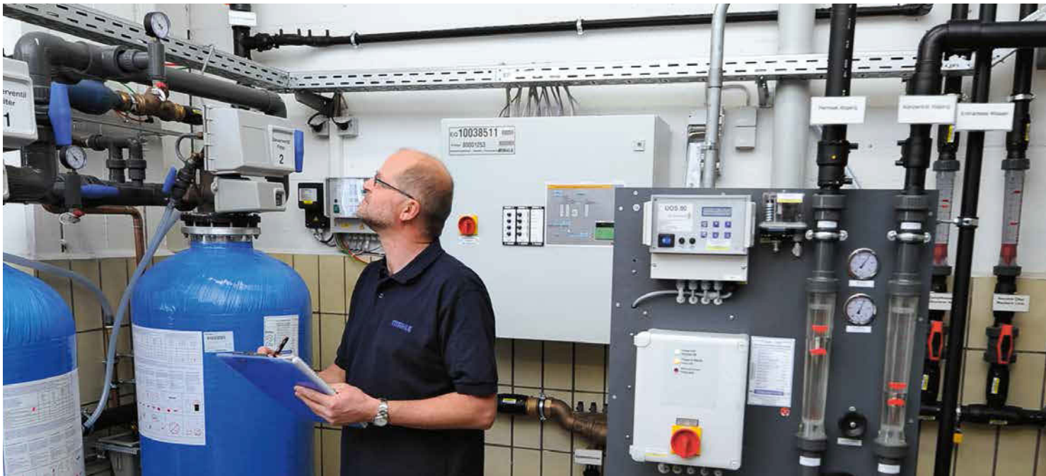
Water treatment in the central cooling water supply of the Mühlacker/Germany plant is carried out using a new environmentally friendly reverse osmosis system.
