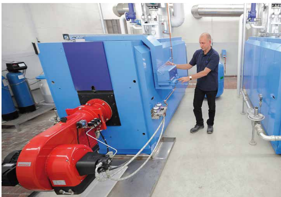
Energy consumption, particularly for heating and air conditioning systems, offers considerable savings potential.
